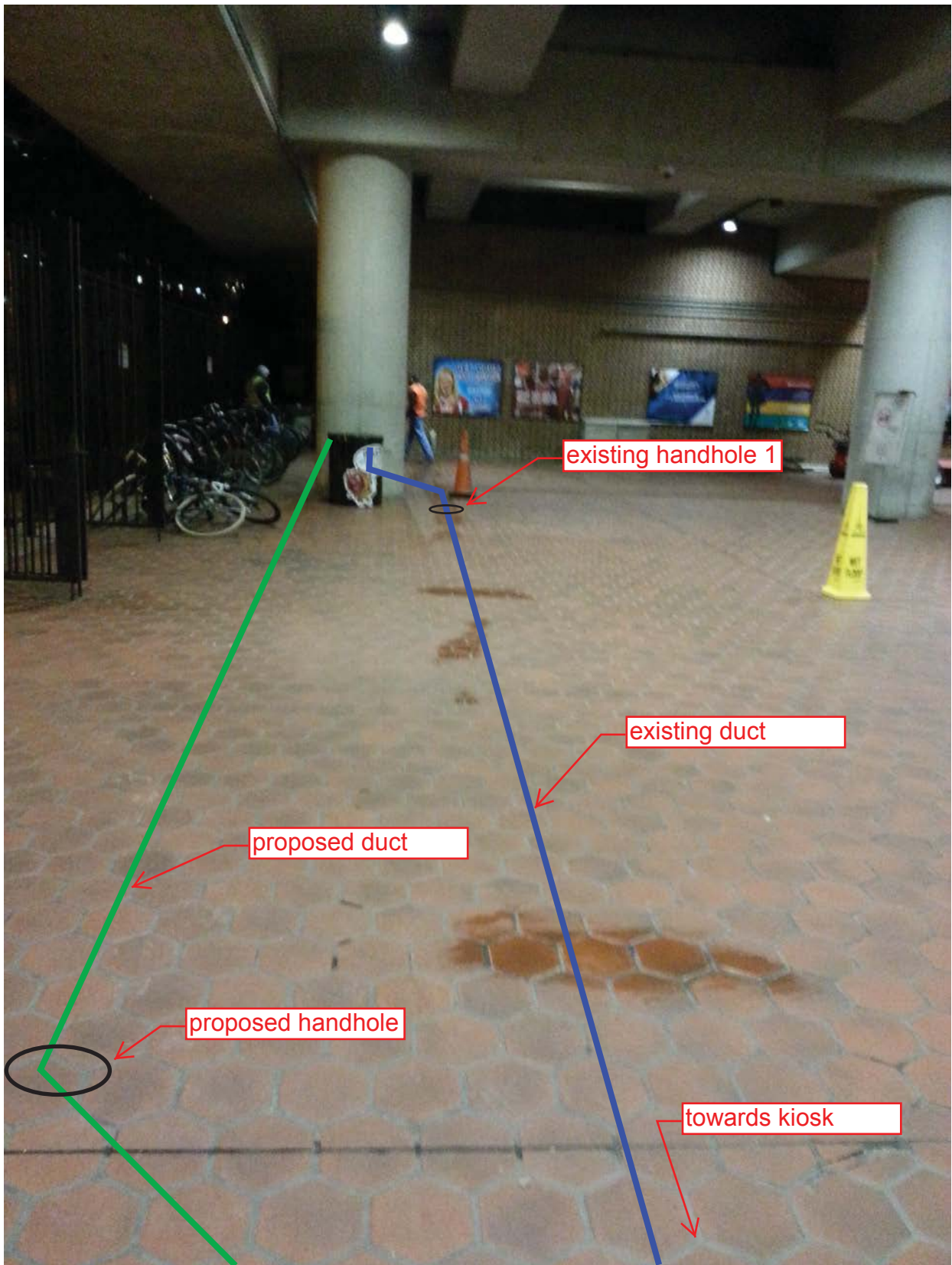
Photo #2 – C13 King Street South: Existing and proposed duct runs towards backrooms
